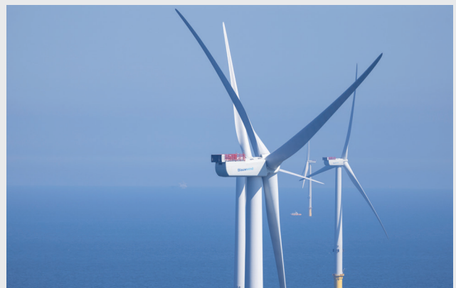
Wind turbines at the Borssele III & IV offshore wind farm in the Dutch North Sea. Source: Blauwwind
