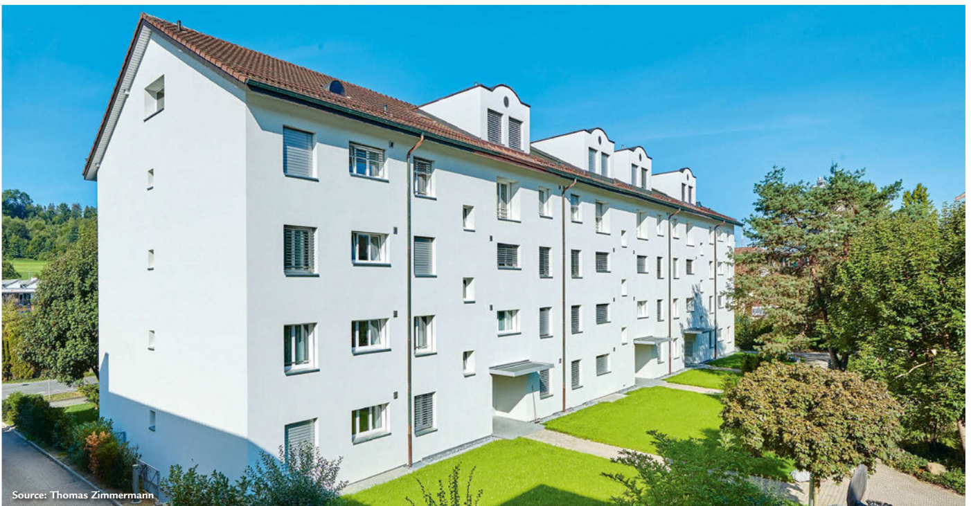
Complete façade refurbishment and replacement of heating system reduce energy and ancillary costs
